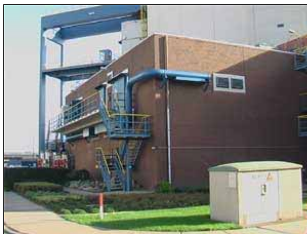
Figure 3. Air intake of bunkered diesels.
