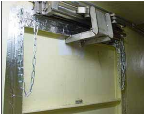
Figure 2. Remotely opened explosion hatches.
