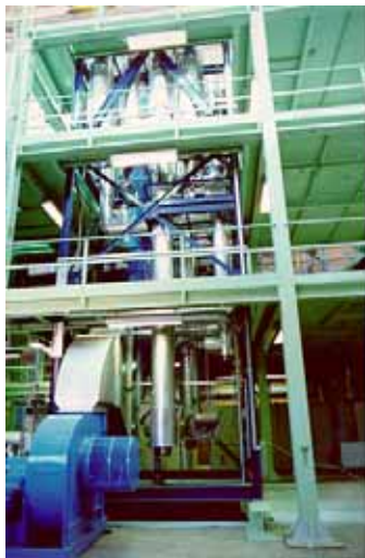
Figure 3: HE-FUS3 helium loop, IHX mock up testing, ENEA Brasimone (Italy)
