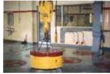
High active waste storage
