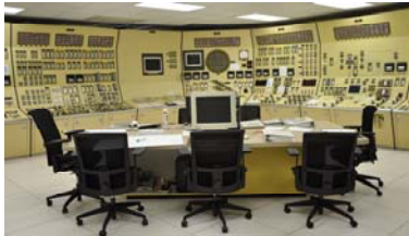
Figure 2 - Nuclear Reactor Control Room Simulator
