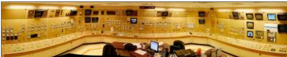
Fig 1: 1300 MW nuclear station control room
