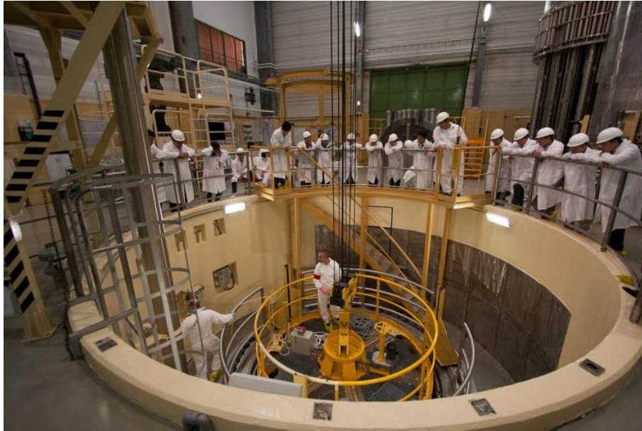
Fig. 6: Demonstration of lifting the reactor internals in Maintenance Performance Improvement Center of Paks NPP
