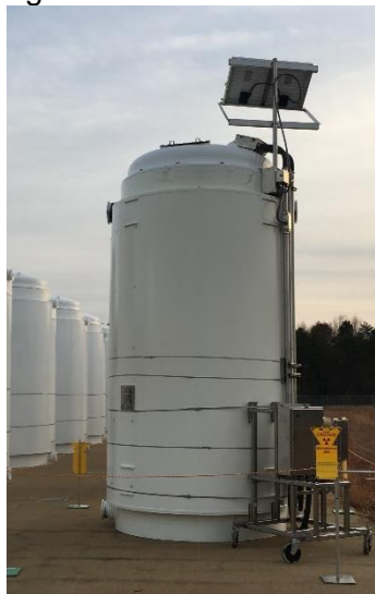
Figure 4. HBU Research Project Cask at North Anna ISFSI
