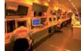
>> MELOX control room
