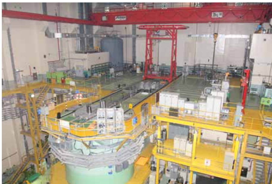
Figure 1 View of the reactor hall
