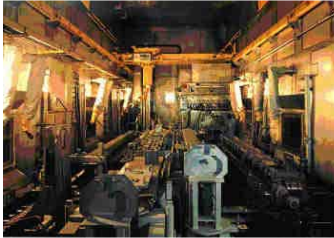
Fig. 3 Hot cell of the pilot conditioning plant
