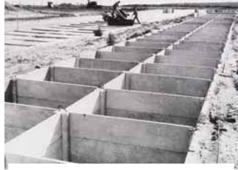
Figure 2: concrete disposal cells
