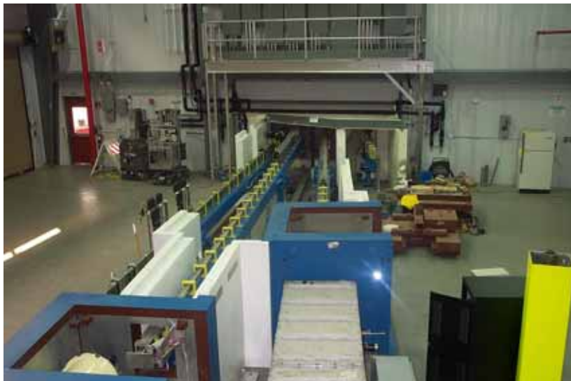
Figure 4: Guides installed in HB-4 Guidehall
