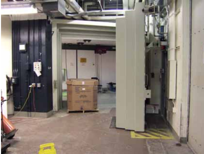
Figure 2: Open Shield Tunnel Door in Beam Room
