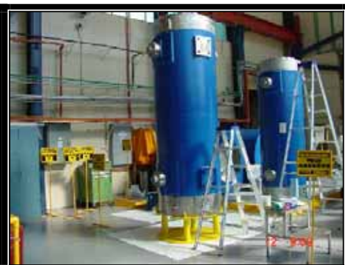
TN 7/2 Cask Loading Preparation Area
