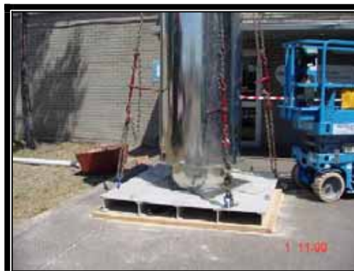
NAC-LWT Cask Loading Area
