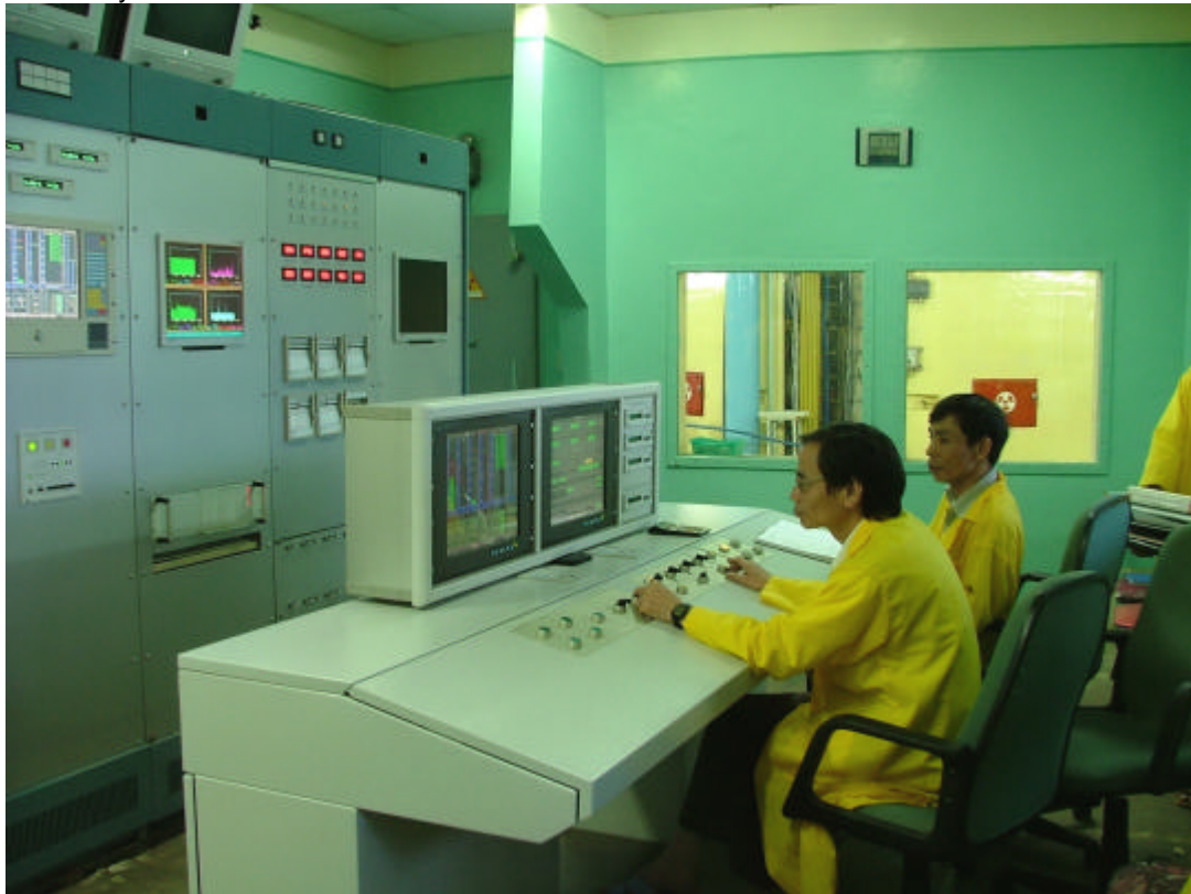
Fig 1. Operation of DNRR with new control system
