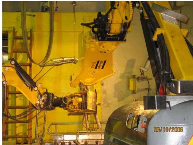
Fig. 1. Cutting elements of loop channels, using remote-controlled robotic mechanisms «BROKK-180" and «BROKK-330"
