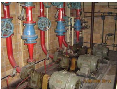
Fig 6. First cooling loop prior the dismantling
