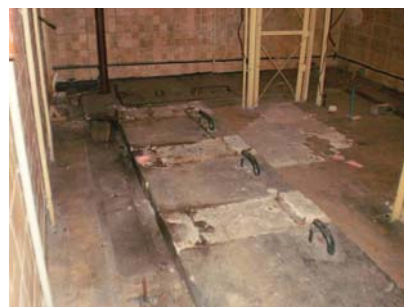
Fig 7. First cooling loop after the dismantling
