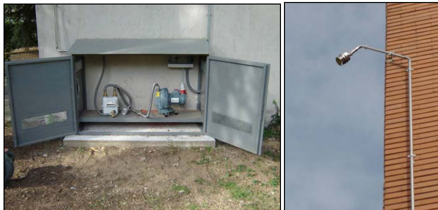
Figure 4 – Environmental air particulate monitoring station and air vent (mounted 5m above ground)
