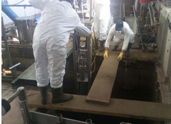
Figure 4. WCCS Installation in Vinca Fuel Storage Basin 4
