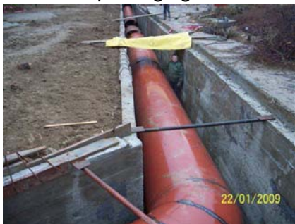
Fig 5. New ventilation pipeline
