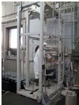
Fig 7. Working platform was brought to the Working platform in the spent fuel storage, where further cutting of the fragment tube with manual cutting device enabled transferring fuel elements into new canisters.
