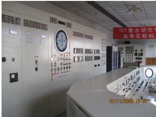
Fig.2: The main control room of HWRR
