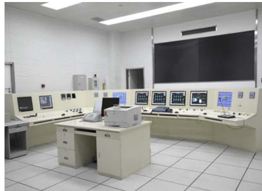
Fig. 3: The main control room of CARR
