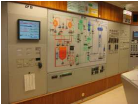
Fig. 9 The control room with old-style panels before the installation on the LSD
