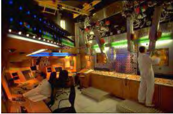
Fig.31: De-storage facility control room © AREVA
