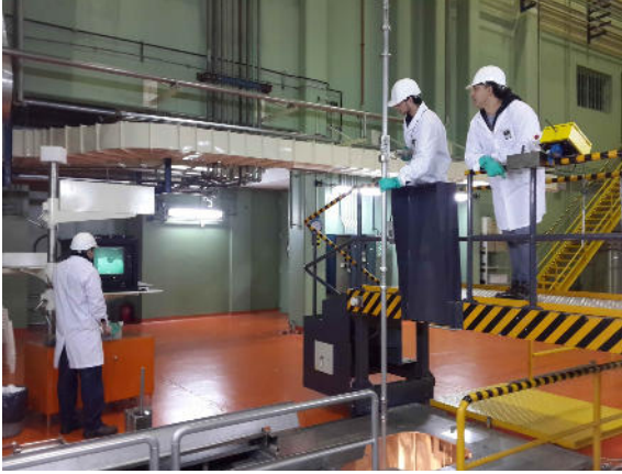
Fig. 6: View of the operator on the mobile platform handling a grappling tool.
