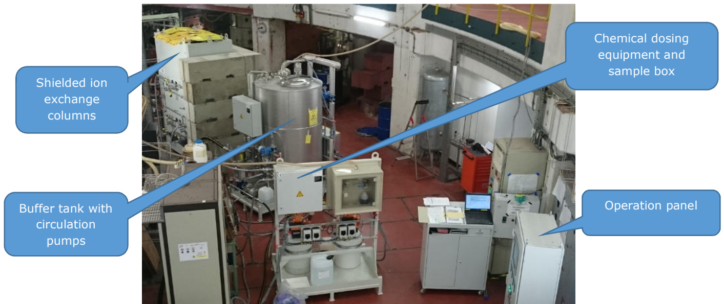
Figure 3: Installation for decontamination in the BR2 containment building
