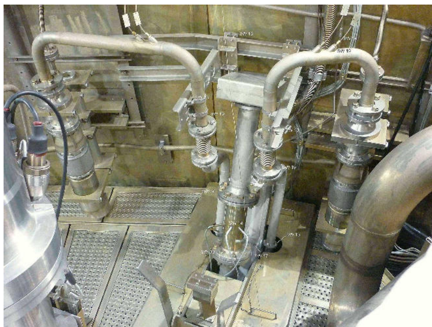
Fig 1. The installations of the converter facility inside the reactor pool
