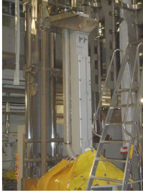
Fig 7. Outer duct in the rack in the reactor hall with shieldings
