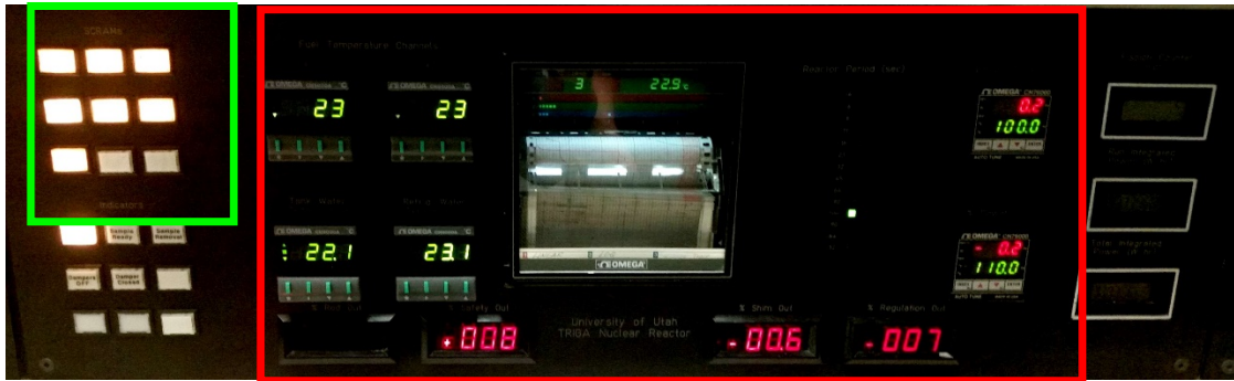
Fig 4: UUTR Central Panel
