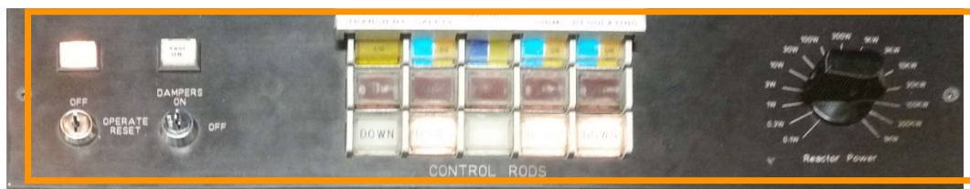
Fig 6: UUTR Lower Central Controls
