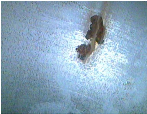
Fig. 3: Affected inner surface of the thimble.
