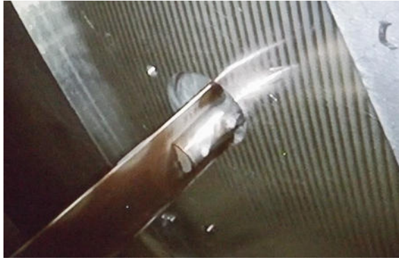
Figure 6: CCTV image from below the Interface Plate confirming CR blade located in recess to ensure correct cut position.
